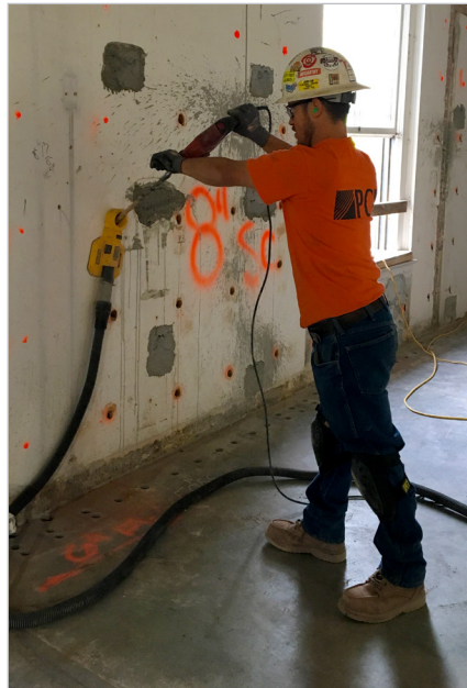
Drilling at the required 22.5° angle to install epoxied rebar before adding shotcrete to URM wall.
