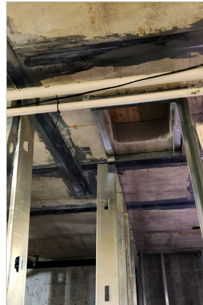
FRP laminates used for diaphragm strengthening (shown), with clips on stud walls (not shown).
