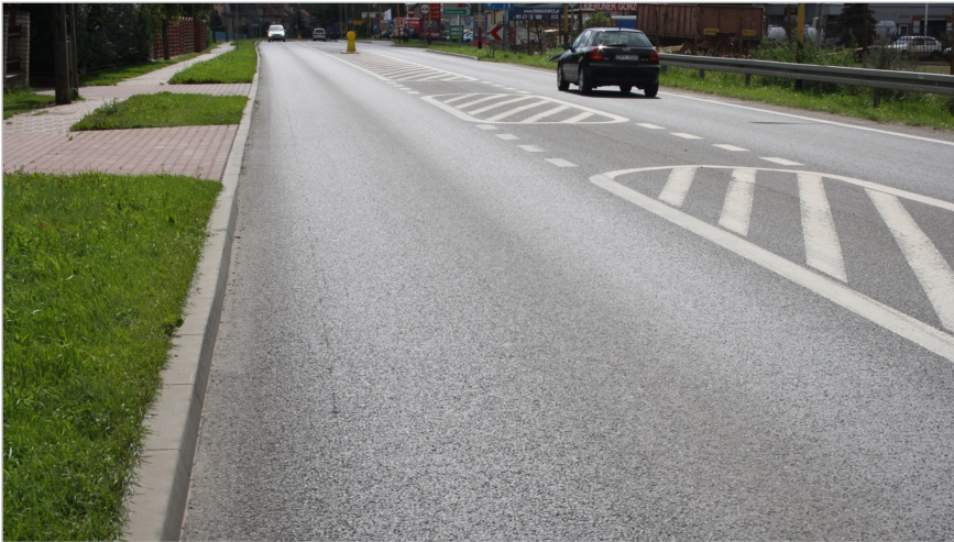
Simpson Strong-Tie worked together with the road administrator to come up with a long-term, durable solution.
