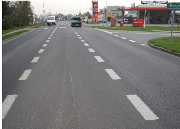
2014 — Even eight years later, there is still no damage to the wearing course and only the longitudinal joint where the two pavement sections were merged is visible.
